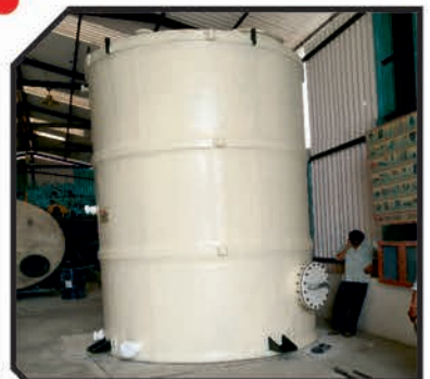
PPGL FRP STORAGE TANK 30KL
